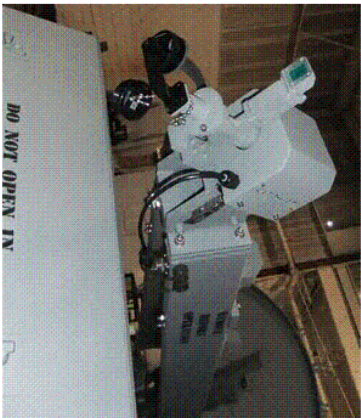
Pol Dangle install RCI P# FP-P2_PL_DNGL2 FP-P2_PCBL_030 BOX RECP installed on bottom of beam
